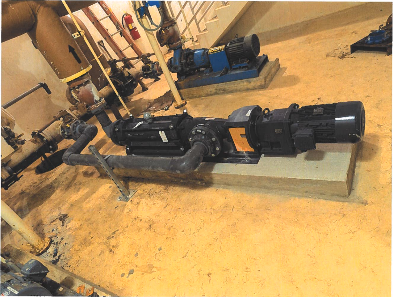
Installed Sludge Pump
