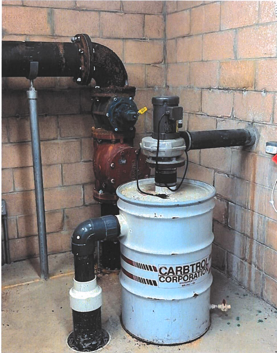
Carbon Cannister Inside Station 73
