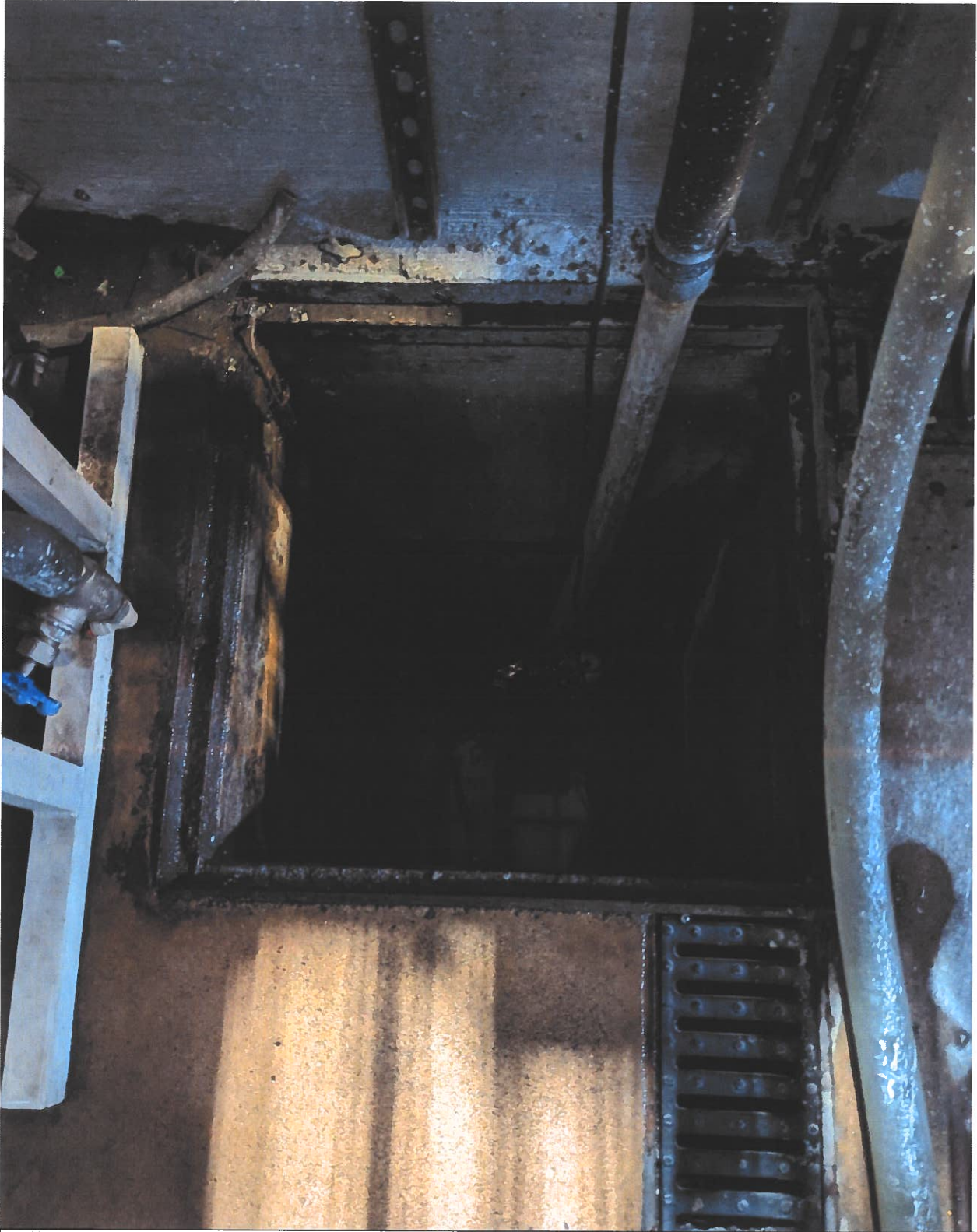
Floor Drain Sump with Discharge Piping Going into Waste Tank
