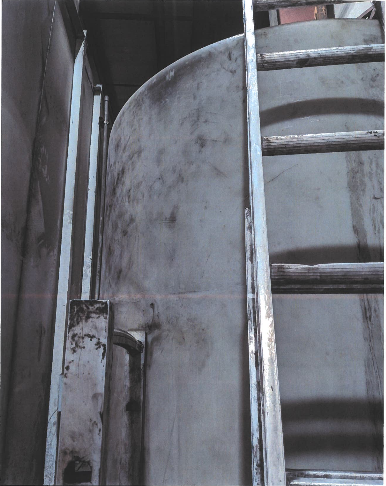
Waste Tank Inside Containment Area
