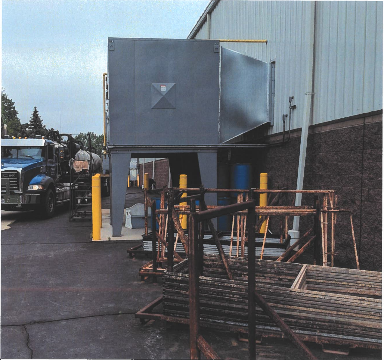
Waste Hauling Company with Tanker Connected and Pumping to Remove Waste Product on May 21, 2024
