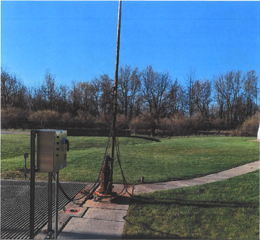
Post Aeration Pump
