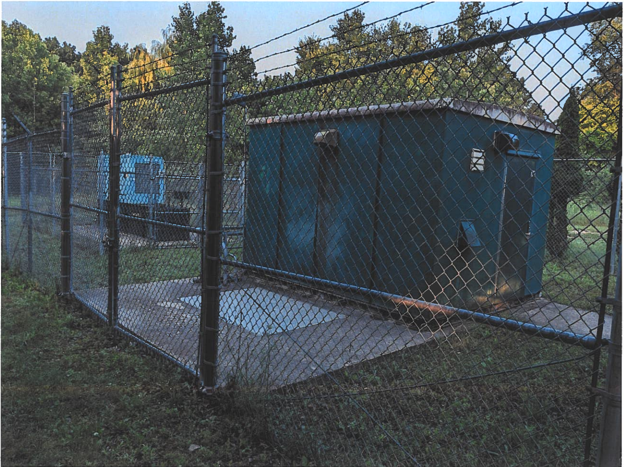
Pump Station 74 Located on Tooley Road
