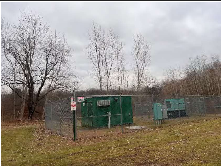
Photo 12. South adjoining and Subject Property, Sewage Pump Station
